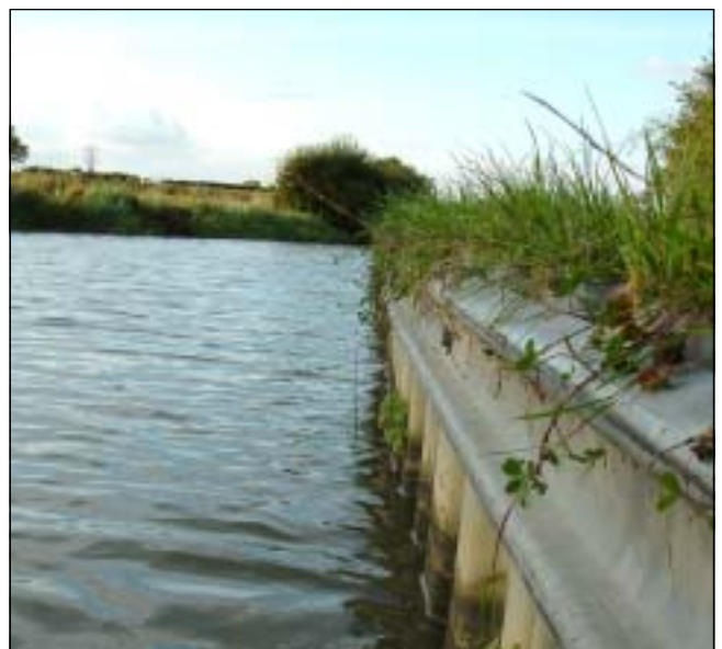
Figure 3. Bumper on galvanised steel piling.
